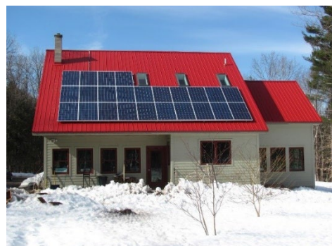
PICTURE 5B-1. RESIDENTIAL HOUSE WITH ROOFTOP SOLAR PANELS
